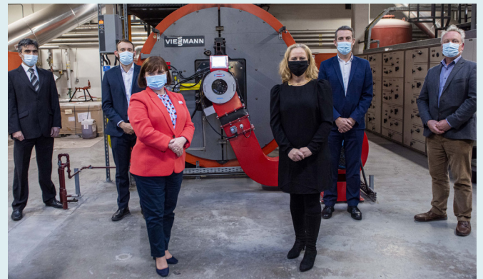
Pictured from left to right at the announcement were Seamus Foran, Head of Project Management Office TUH; Shane Minehane, Head of Business Operations Centrica Ireland; Lucy Nugent, Chief Executive of TUH; Edel Wyse, Director of Carbon & Energy Ireland Fund; Dermot Carter, Director of Finance, TUH and Ciaran Faughnan, Director of Facilities & Estates at TUH
